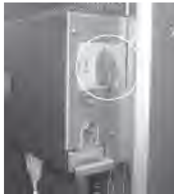
Figure 9: CryoPilot A Main Power Switch
